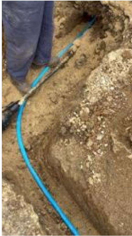
One of two unmarked cables found
