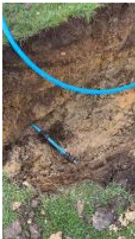
Existing water main to clubhouse
